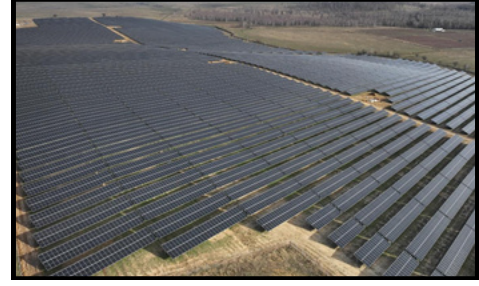
Our Solar Power Plant - Romania
