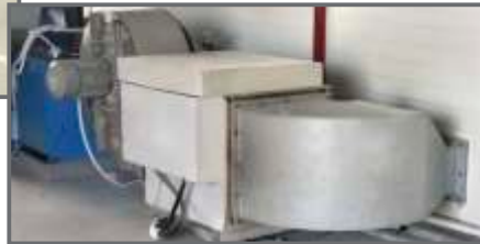
Blower & Heater bank
