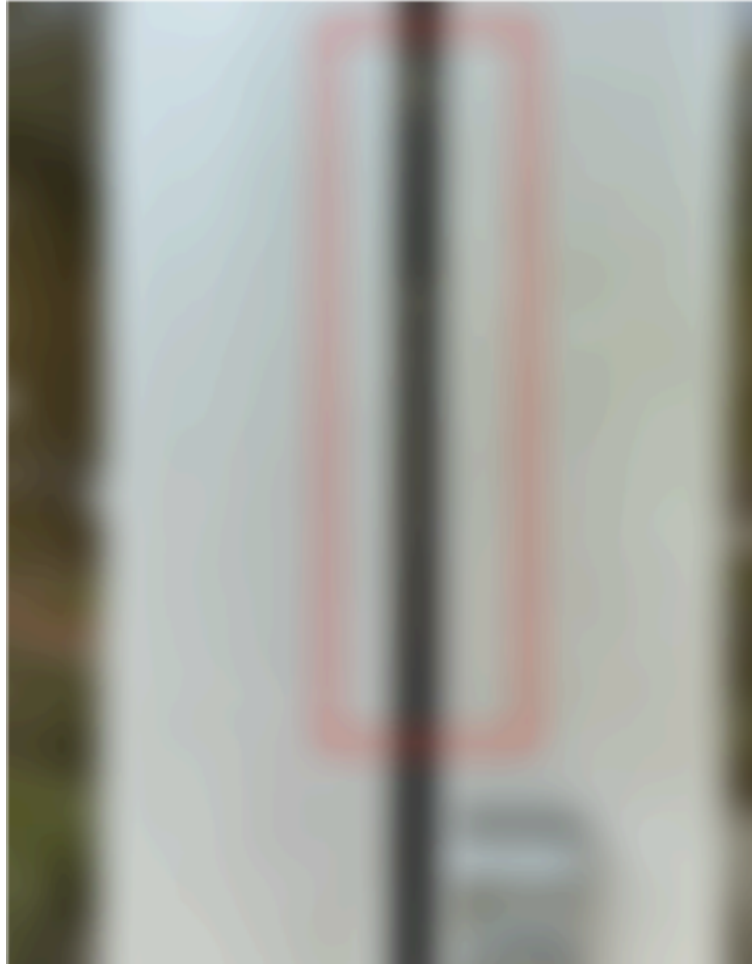
Figure 5: Gap between the entrance doors.
