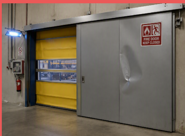
Figure: Damage can impair the door's ability to close and latch reliably. Fire doors should be protected against impact damage from forklifts or other vehicles.
