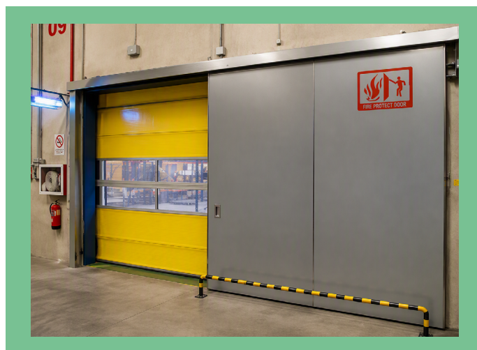
Figure: Fire door equipped with impact protection to prevent vehicle-related damage.
