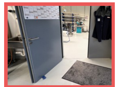
Figure: Blocked fire doors
