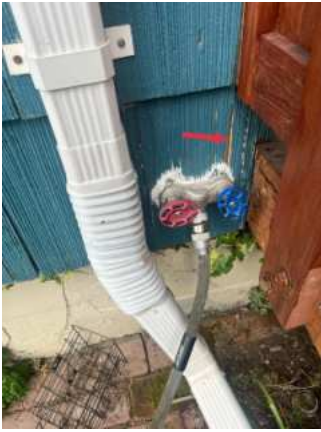
Image 1.10.1 Cracked siding above hose spigot.
