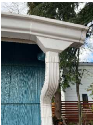
Image 2.6.1 Gutter at downspout with noticeable sagging.
