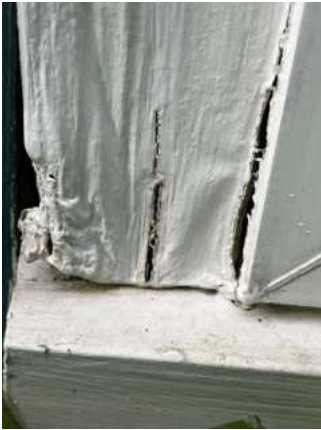
Image 1.2.1 Rot present on basement window trim along south facing wall.
