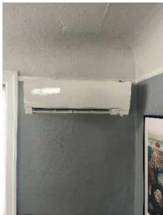
Image 4.5.1 Evaporator unit in living room
