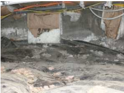
Image 7.L.1 Portion of crawlspace inaccessible because of noticeable rodent debris.
