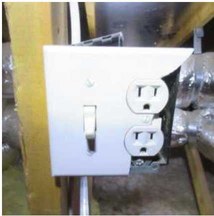
Image 3.8.1 Broken Outlet Cover
