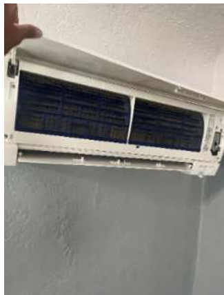
Image 4.5.2 Filters need cleaning
