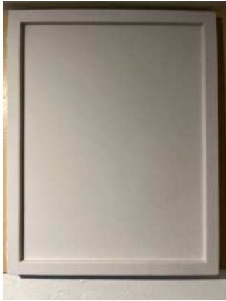
Image 7.1.1 Crawl space entry door, not insulated.
