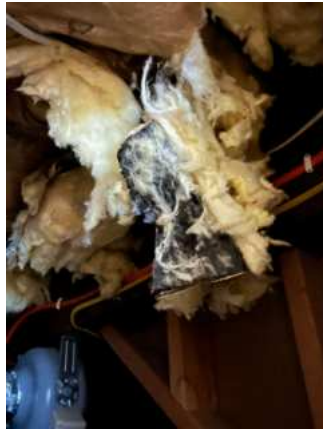
Image 7.1.2 Example of falling insulation in crawl space.
