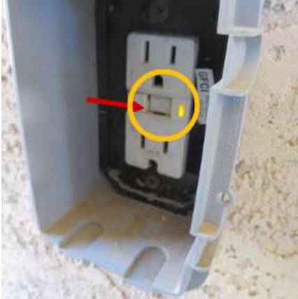
Image 3.6.1 Broken GFCI Test Button
