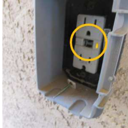
Image 3.6.2 Broken GFCI Test Button
