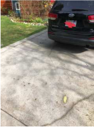
Image 1.8.1 Cracking in driveway
