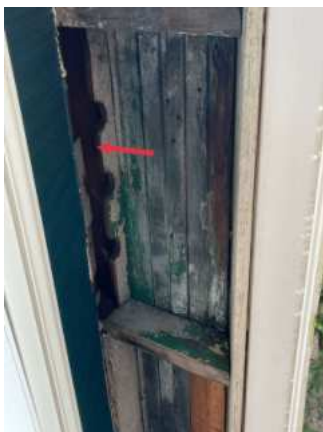
Image 1.7.1 Soffit vents missing open exposure to attic. Broken bird blocking.
