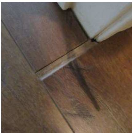
Image 6.1.1 Hardwood Flooring Gap - Master Bdrm Entry
