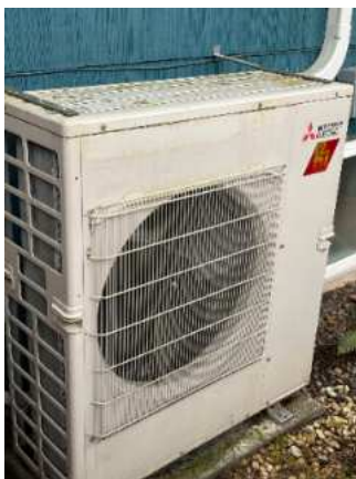
Image 4.2.1 Condenser unit located on North facing wall
