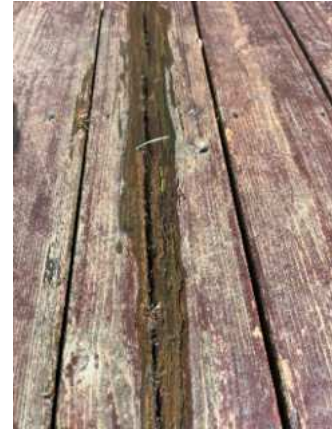
Image 1.4.3 Rot from water penetration. Deck board should be replaced.
