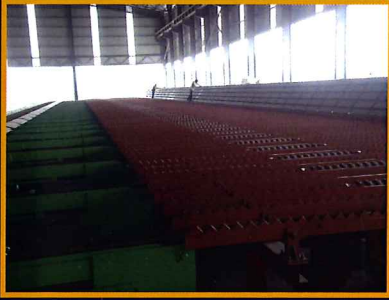
Automated Cooling Bay
