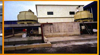
Transformer Building & Water Cooling System
