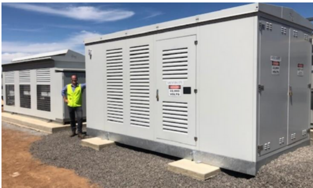
Solar HV Skid Three - 1.217MW
