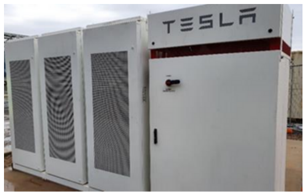
Tesla 500kW/1232kWh Battery Pack
