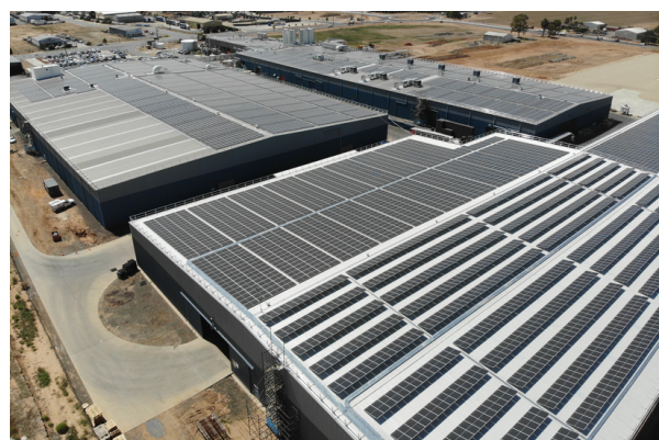
Solar PV - Ariel View 2
