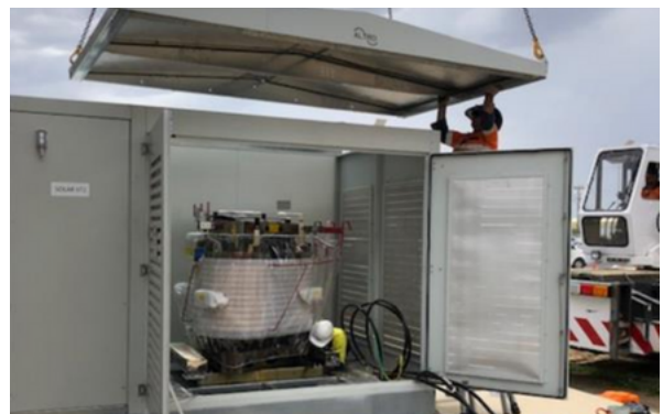
Solar HV Skid Two - 1.282 MW
