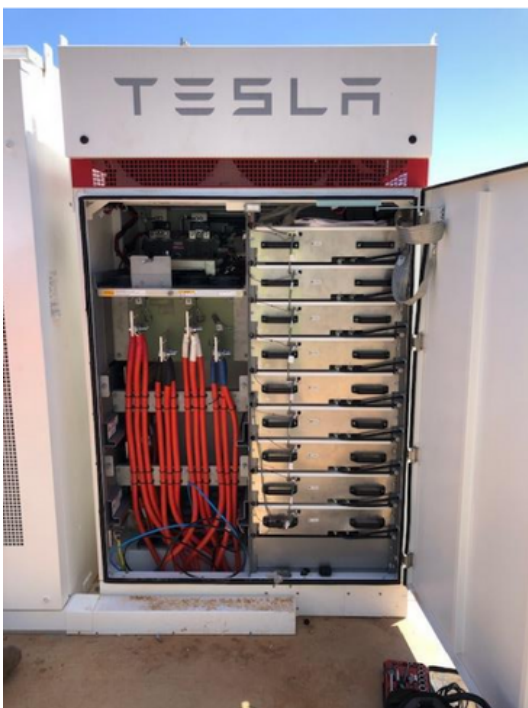
Battery 500kW Inverter
