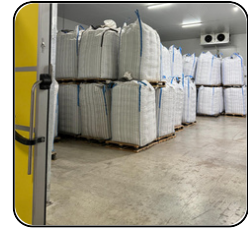
Inside the Cold Storage Room
