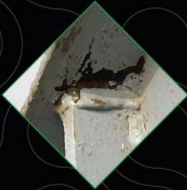
Under film corrosion
