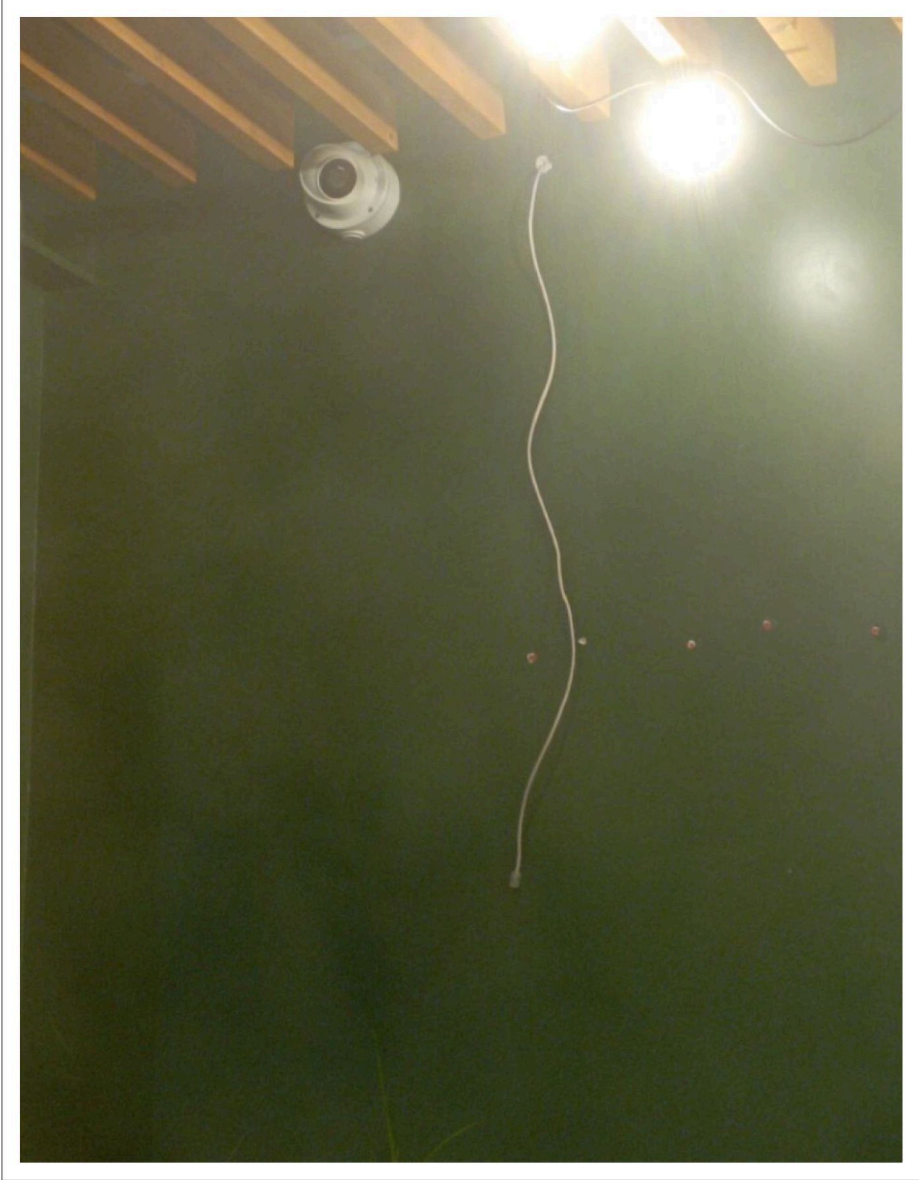
Figure 1: Real pic of an Ethernet cable leaved in a public area of a plant.
