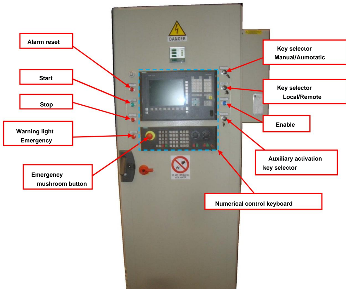
Figure 7 - General electrical panel
