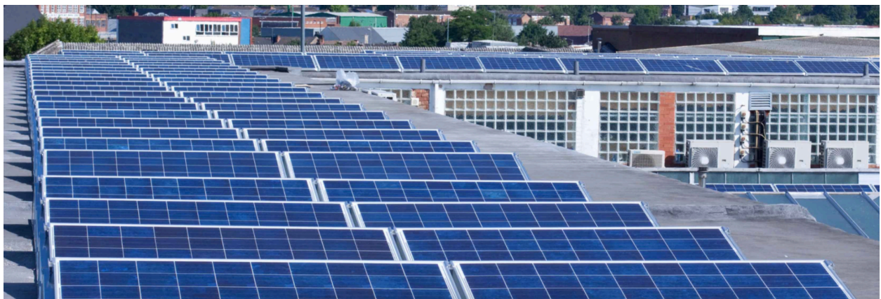
Figure 3. Rooftop Solar Array Concept. (Zeoluff)
