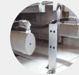
Hydraulic Power Unit
