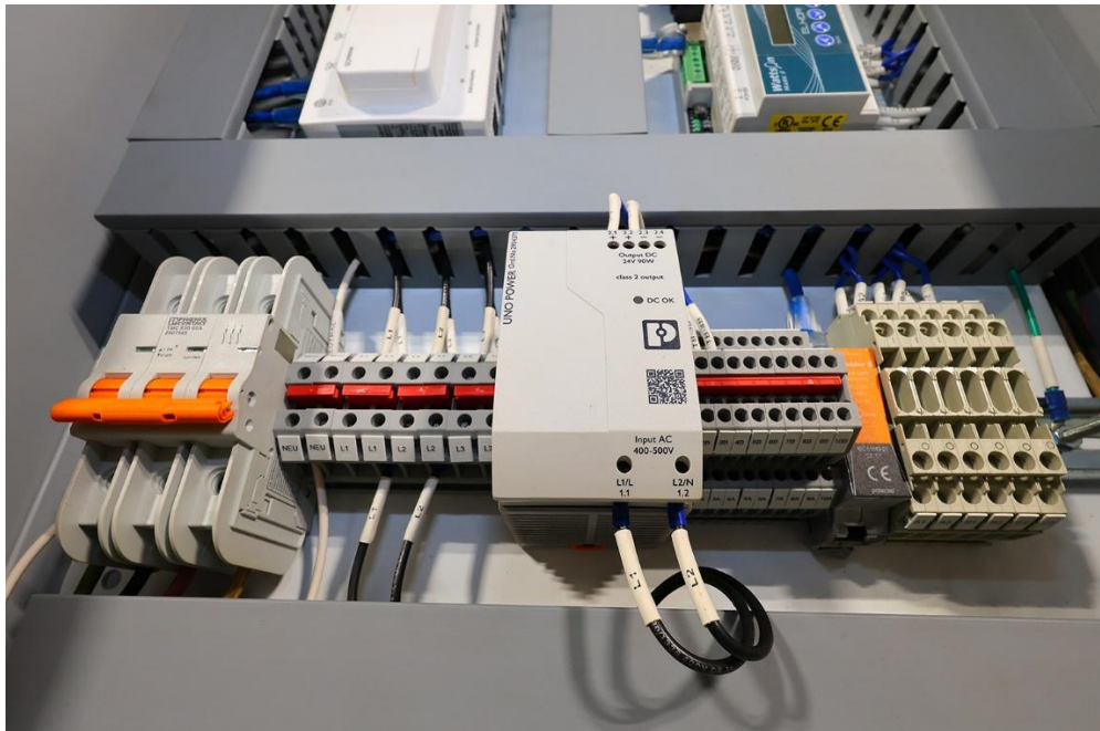
Figure 5 – Focus on 3-Phase Power Conversion to 24VDC and Signal Input Stage
