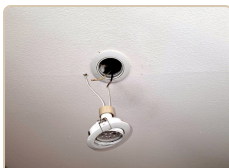
Loose downlight, bare wires
