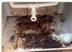
Sink cabinet: rusted base
