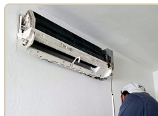
AC unit opened for cleaning
