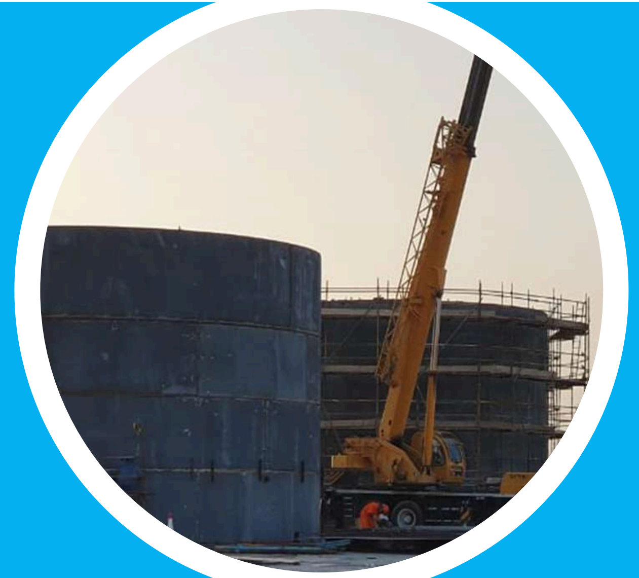
Manufacturing of API 650 Oil Storage Tanks at KIZAD for Aden Power Plant in Yemen Client: Petromasila / GE
