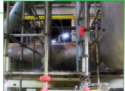
Initial appearance of the line with the high pressure leak
