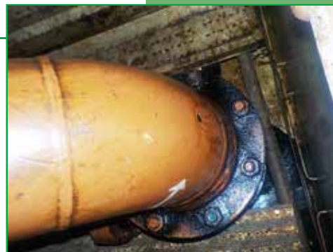
Initial appearance of the line the hole near the junction
