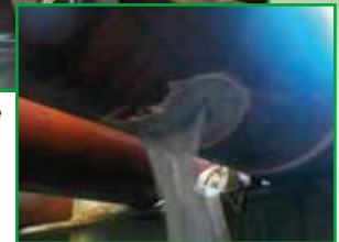
...and the leak
