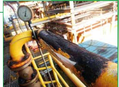
Initial appearance of the line with severe corrosion
