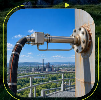
STACK EMISSION MONITORING
