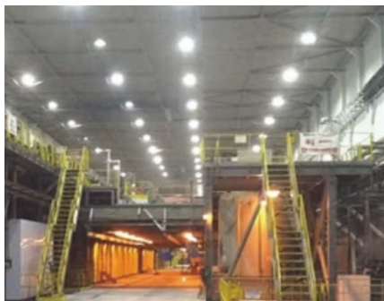
Steel Mills: Capable of withstanding harsh environments and high temperatures.
