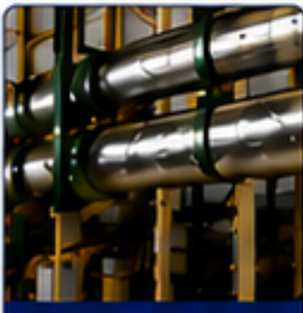
PIPE INSULATION WRAP
