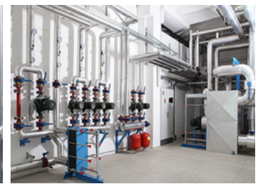
Site, City Heating Applications
