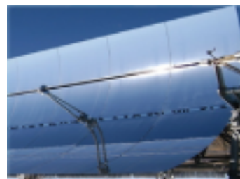
Solar Collector and CSP Applications
