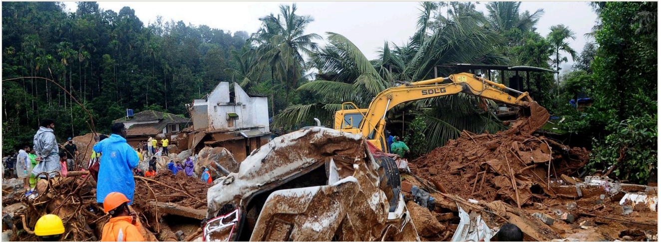
POST LANDSLIDE ASSESSMENT, WESTERN GHATS. DEBRIS EXTENT AND STRUCTURAL LOSS RECORDED FOR RELIEF AND FOR THE RECORD
