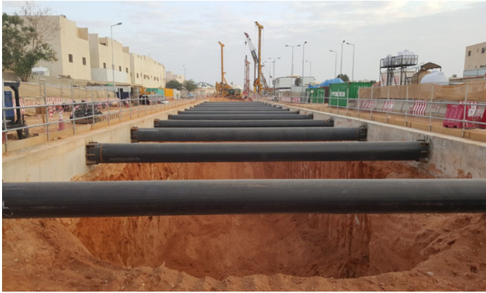
Riyadh Metro, KSA
