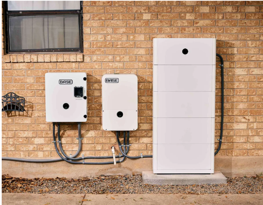
A Base Power battery storage system. Photographer: Matthew Johnson for Bloomberg Businessweek
