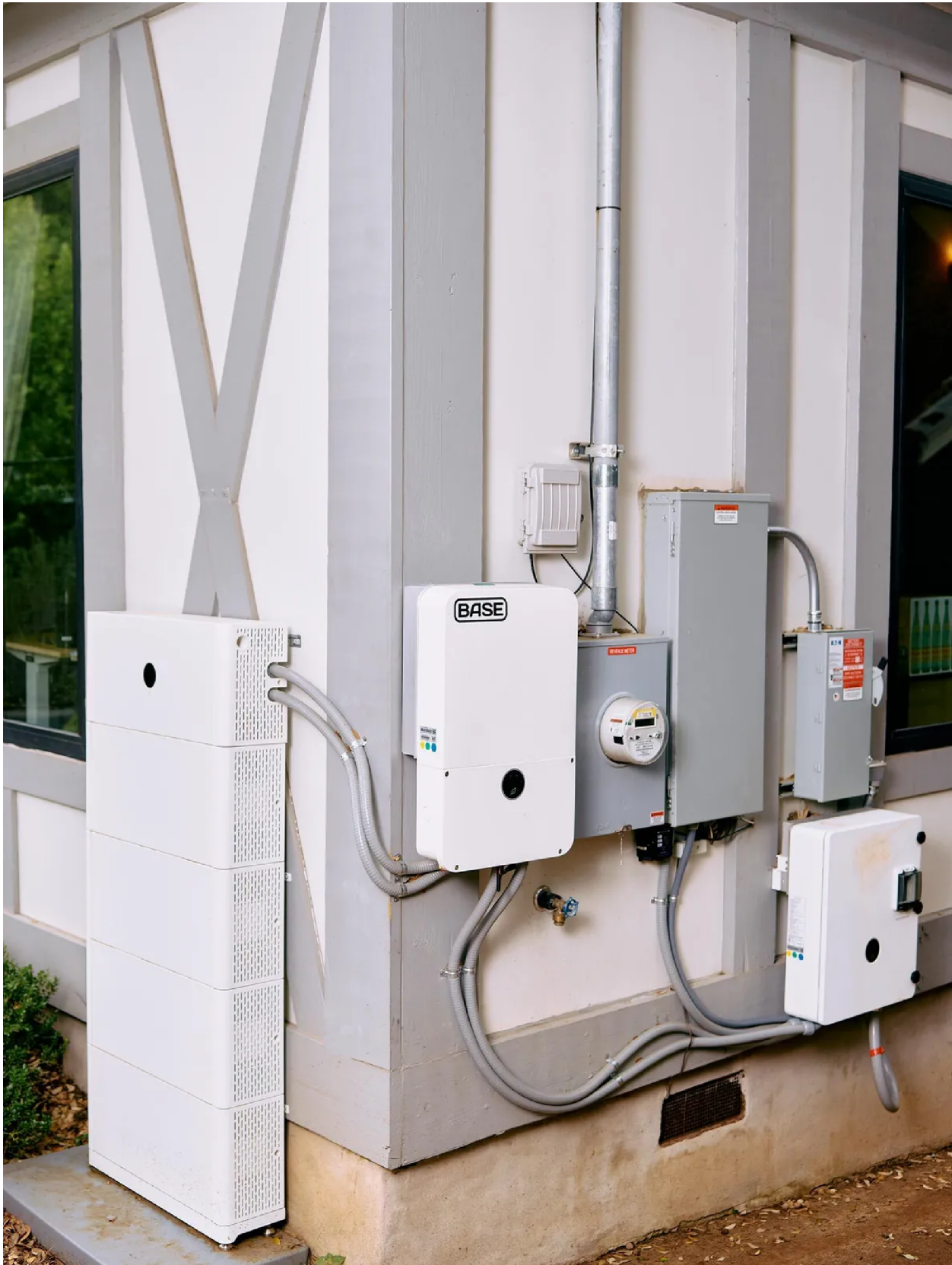
A Base Power system will cost a homeowner $2,000 for equipment and installation. Photographer: Matthew Johnson for Bloomberg Businessweek
