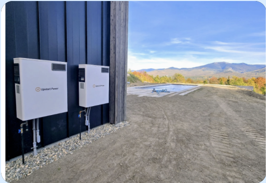
Two Redde units, wall-mounted alongside Trevor's existing solar and battery system in the White Mountains.
