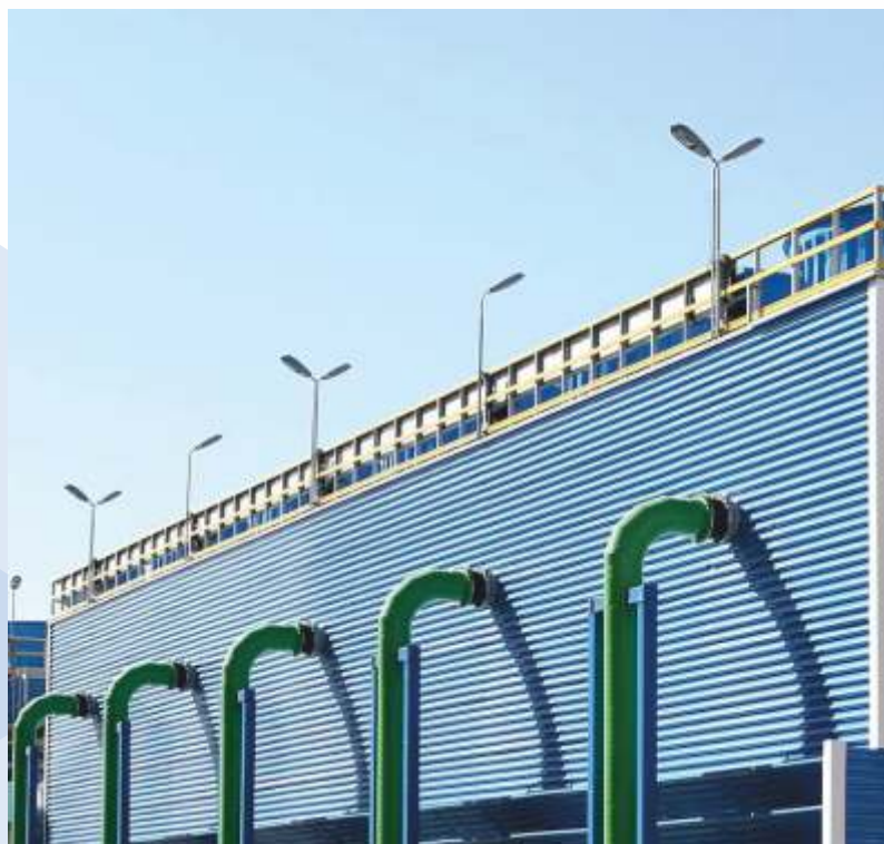
COOLING TOWER AREA
