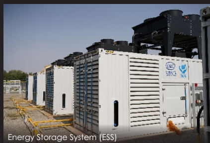
Energy Storage System (ESS)
