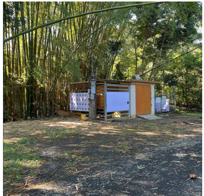
Pumping station for the Corcovada Community Water System.
